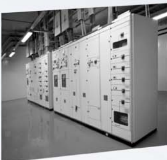
Communication (Electronic exchanging equipment)
